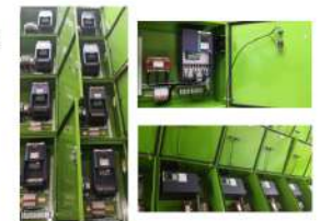
customized solar pump control panel
